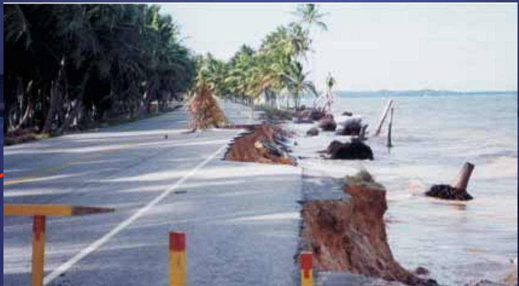
Destruction of roads.
